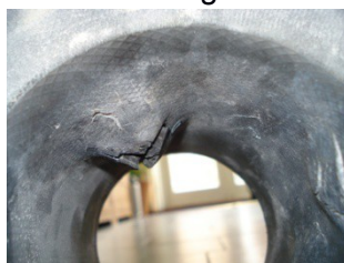
Damages of rubber in flange
