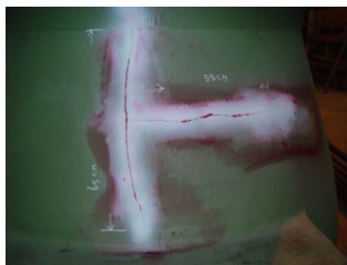
Crack in pump
