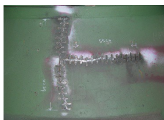
Crack in pump partly repaired
